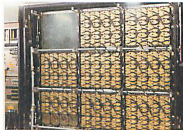
Liquid Cooling Modules
